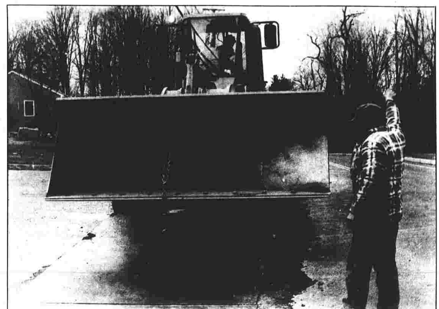
WORK IN PROGRESS — Claude Goupil of East Hartford guides the operator of a front-end loader as he lowers a plate into place on Vernon Street where a new Connecticut Natural Gas line is being installed by the Disenza Construction Co. of West Hartford. The line will serve the large Meadowbrook subdivision of homes on the Manchester/Vernon town line. The subdivision was approved by the Planning and Zoning Commission after Vernon Street had been reconstructed.
